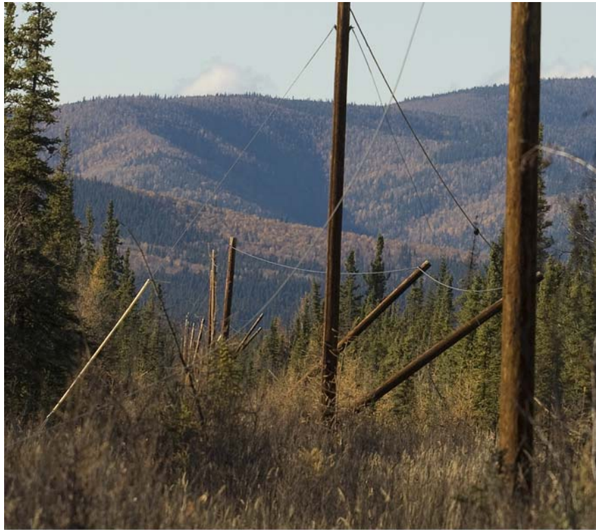
These are drunken power poles. Permafrost melt does not discriminate.
